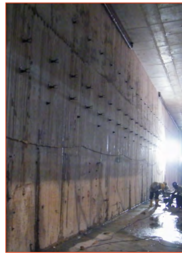
Photo to show wall cast with Cementaid HPI waterproofing system speeded up construction process.
