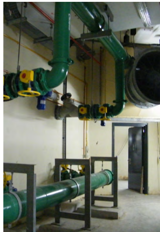
M&E pipes go through the CALTITE wall at Concourse Level with less disturbance and easy detailings.
